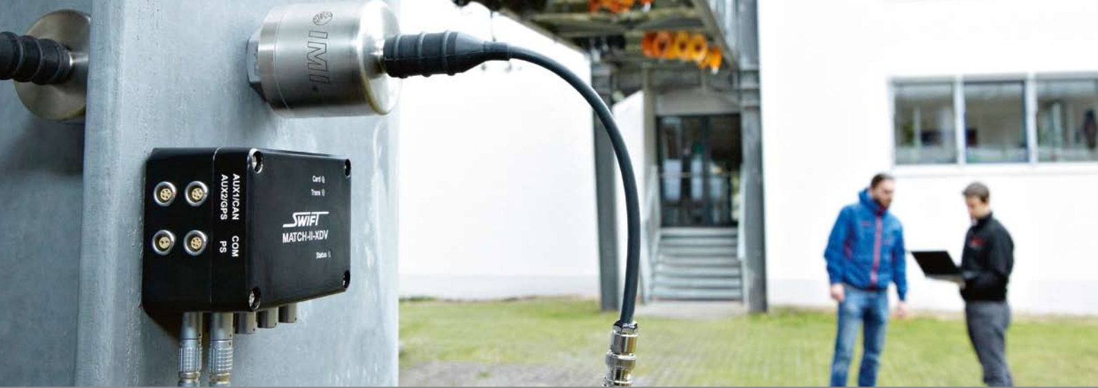
Test des entwickelten Systems an einer Brücke. Test of the developed system at a bridge.
